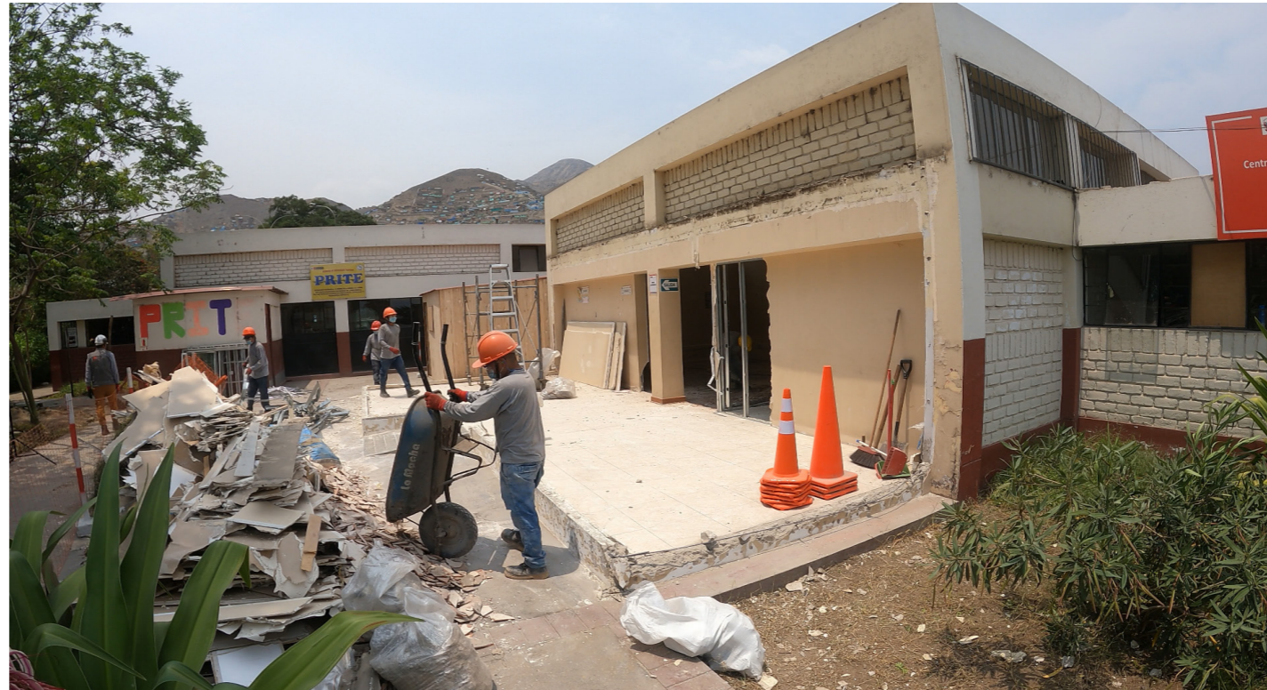
Improvement work at the Comas headquarters of the Alegra center located in Lima Norte.
